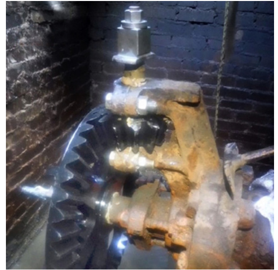
A post-rehabilitation shot of a 36" critical division valve that was inoperable for over 30 years.
